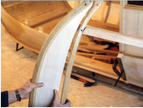
Fitting the quarter panel in the framing. Background shows one in the coach frame.
